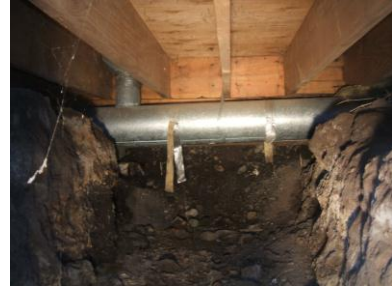
Existing Leaky, un-insulated forced air heating distribution system
