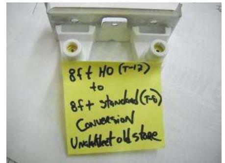
Retrofitted std 8' fixture lamp holders
