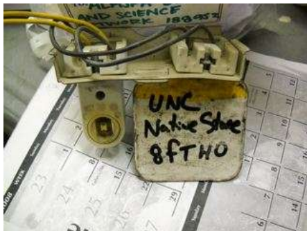
Existing older HO fixture lamp holders
