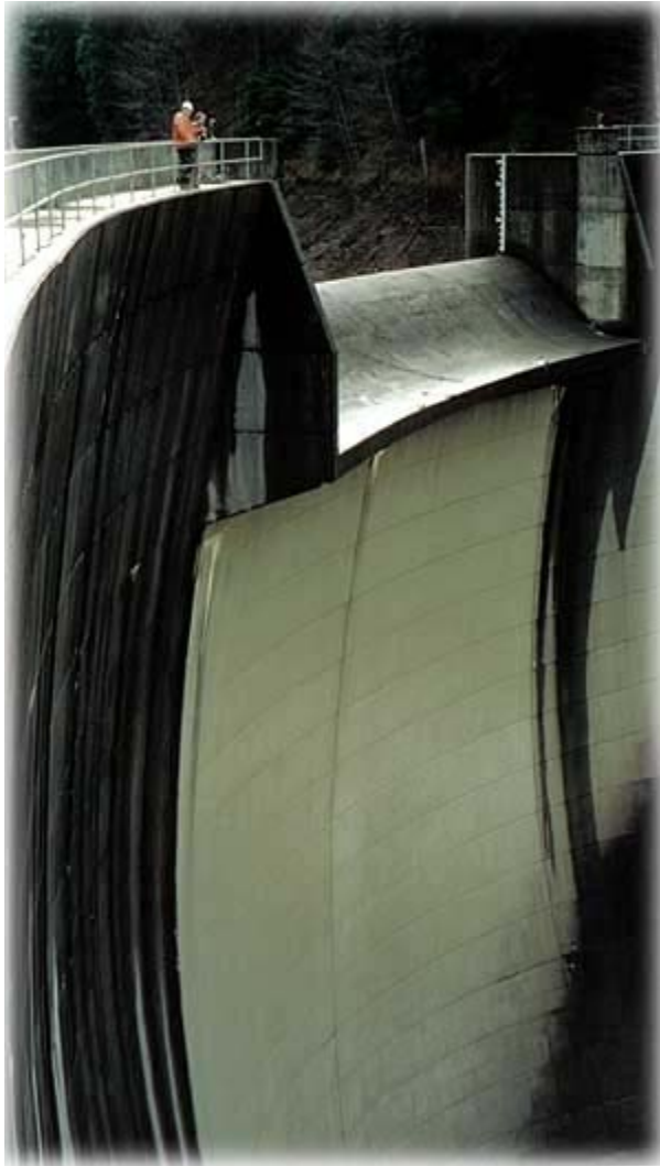
The Swan Lake Project is located approximately 22 air miles northeast of Ketchikan, Alaska, on Falls Creek, which drains from Swan Lake to Carroll Inlet on Revillagigedo Island Photo by Mike Martin©
