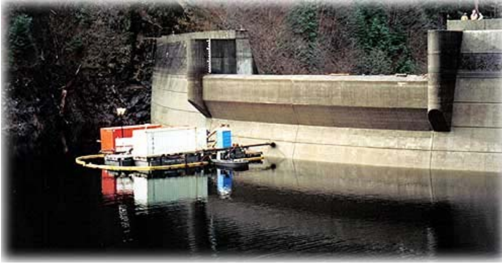
The Swan Lake Project is located approximately 22 air miles northeast of Ketchikan, Alaska, on Falls Creek, which drains from Swan Lake to Carroll Inlet on Revillagigedo Island Photo by Mike Martin©
