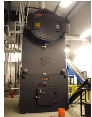
Tok School wood-fired boiler.
