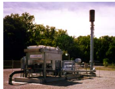
Landfill Gas-to-Energy project in Ft. Wayne, IN showing the gas compressor and backup flare
