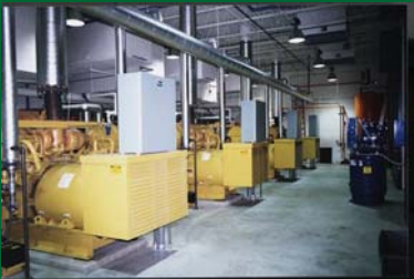
CAT 3616 engines at a LFG power plant in Scranton, PA.
