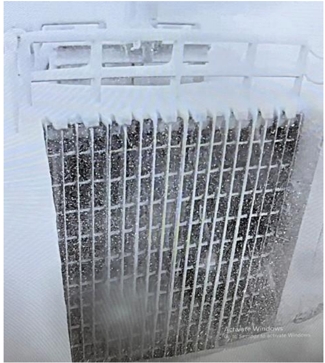
Battle Creek Diversion Inlet Grate
