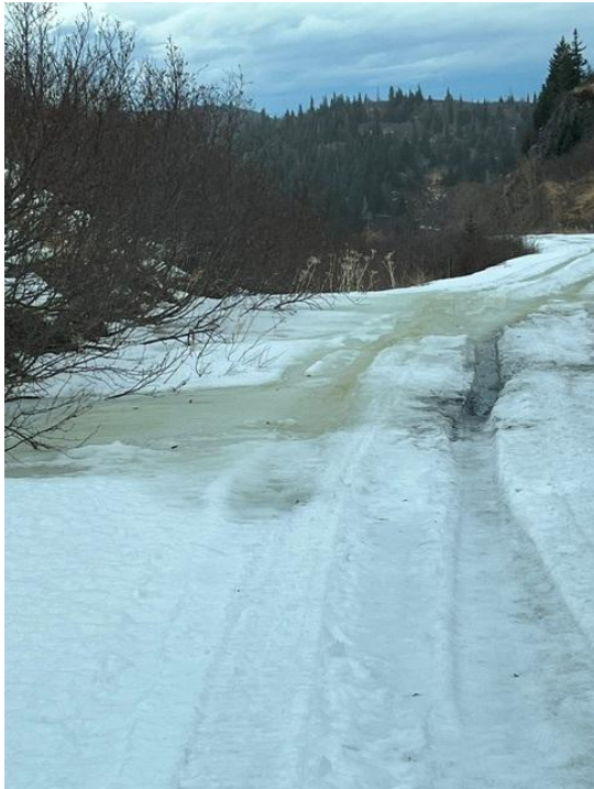
Overflow Ice on Road to Dam
