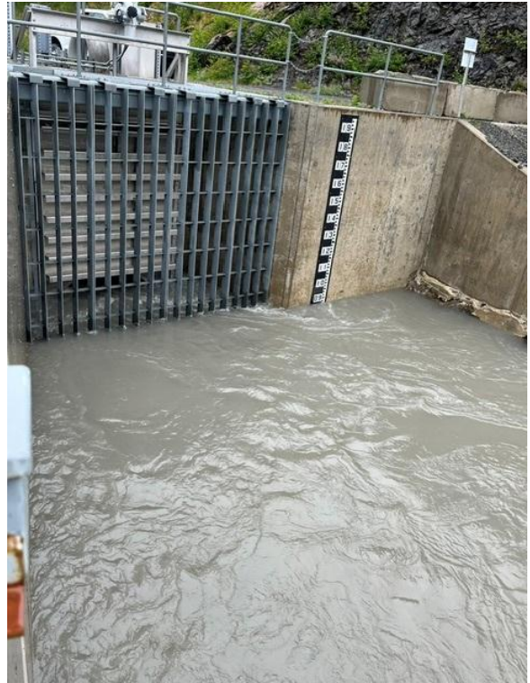
Battle Creek Diversion Inlet Pipe
