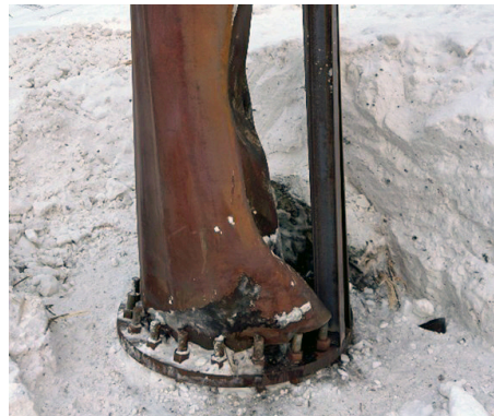
TEMPORARY STEEL BRACE HOLDING TOWER; 14-FOOT DENT VISIBLE
