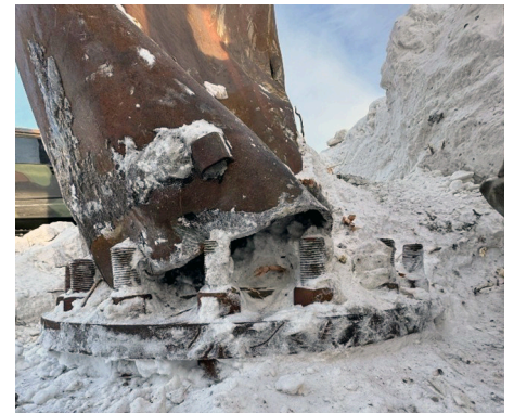
CLOSE-UP OF TOWER PARTIALLY DETACHED FROM BASE PLATE
